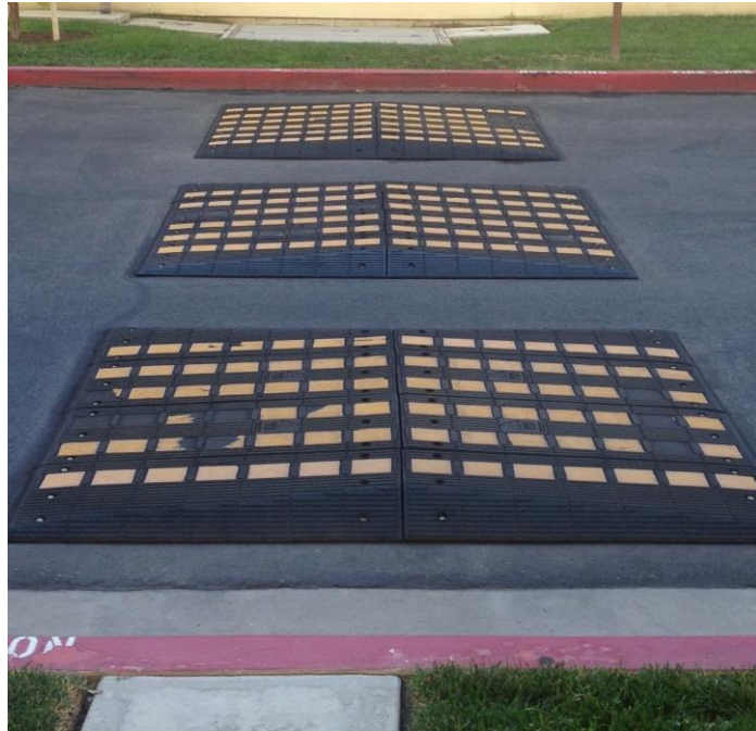
Figure 1: Example of rubber speed cushions installed across a fire lane. Locate the first speed cushion in the center of the street.
