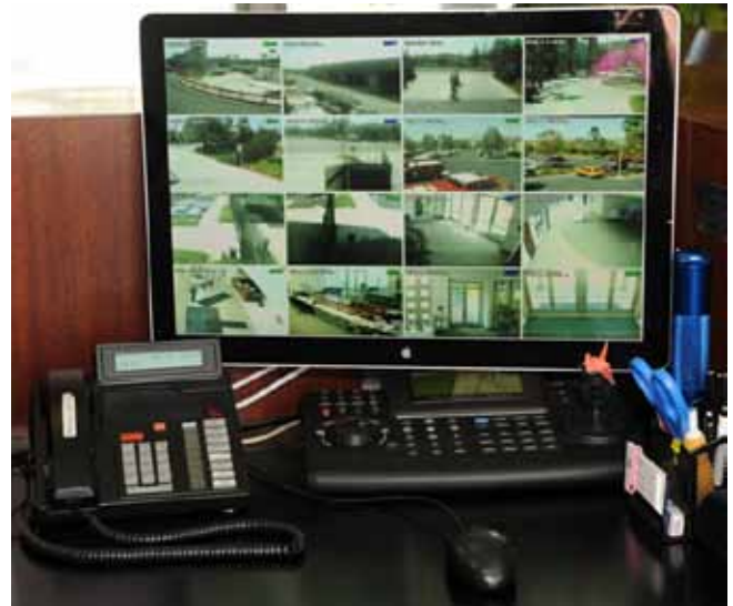
OCFA Security Monitoring System
