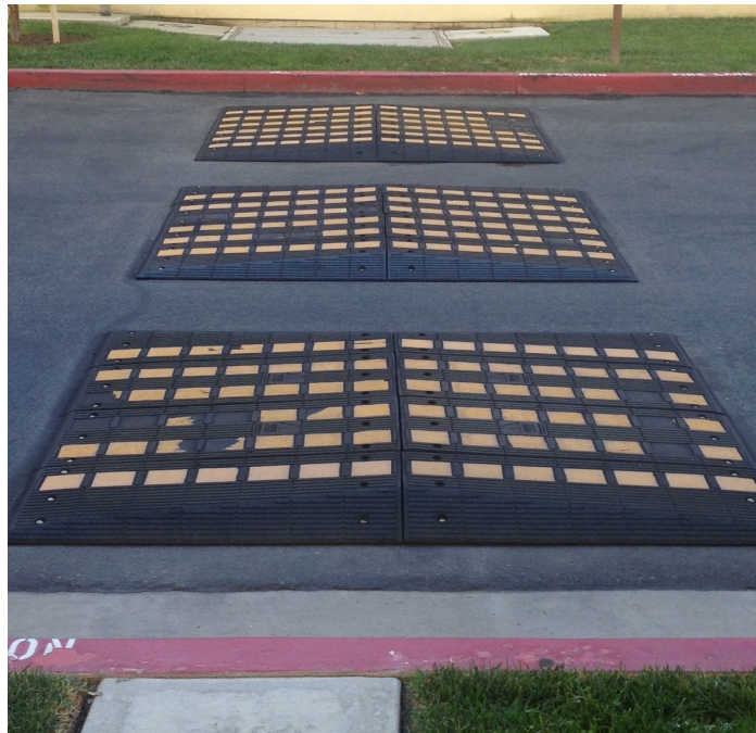
Figure 1: Example of rubber speed cushions installed across a fire lane. Locate the first speed cushion in the center of the street.
